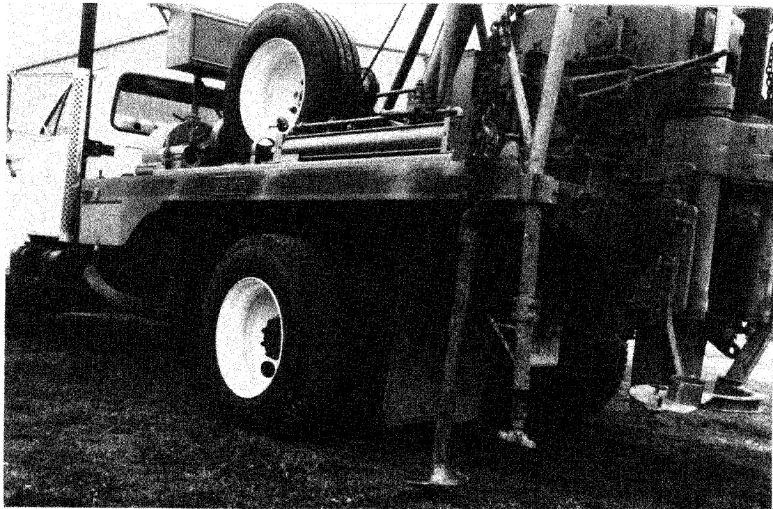
Figure 6-2. Photograph of screw-type earth anchors fastened to the drill rig with load binders to anchor the rig
